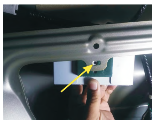
21. Control box installed in the tail gate, with our control box stickers at the back, with a special screw, spring, washer
